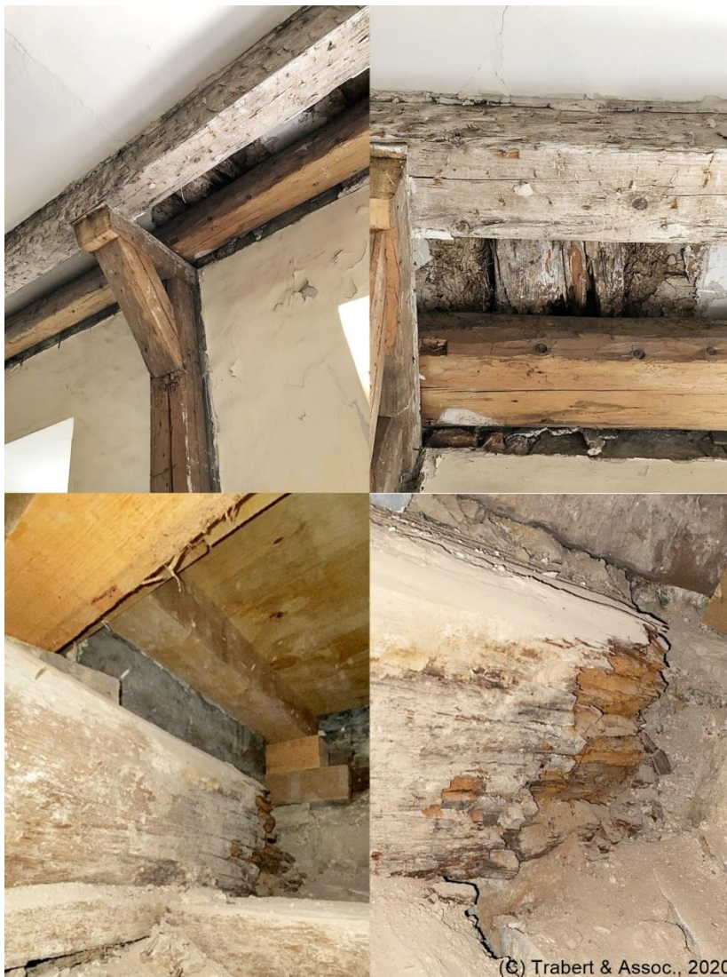
Figure 4: Illustration of state of the timber beams
